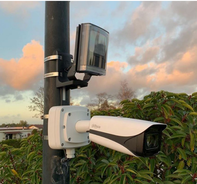
City Surveillance, France.
