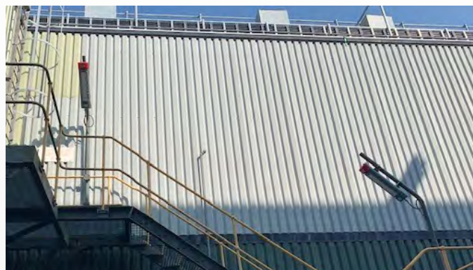
Walkway lighting for Piramal Pharma Solutions
